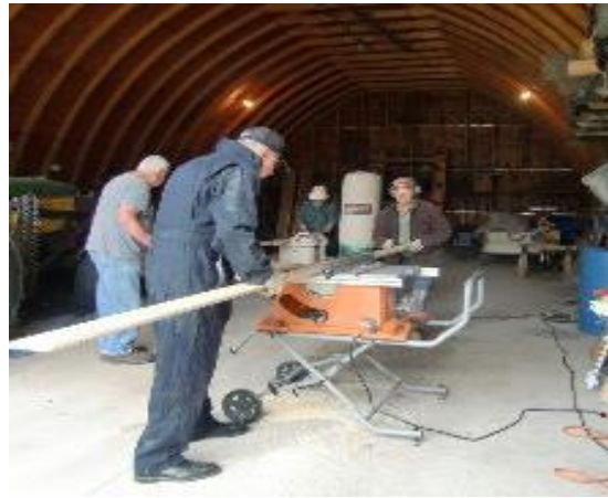
Bill Chimboryk and Bill Rafoss (foreground) cutting a big job down to size.
